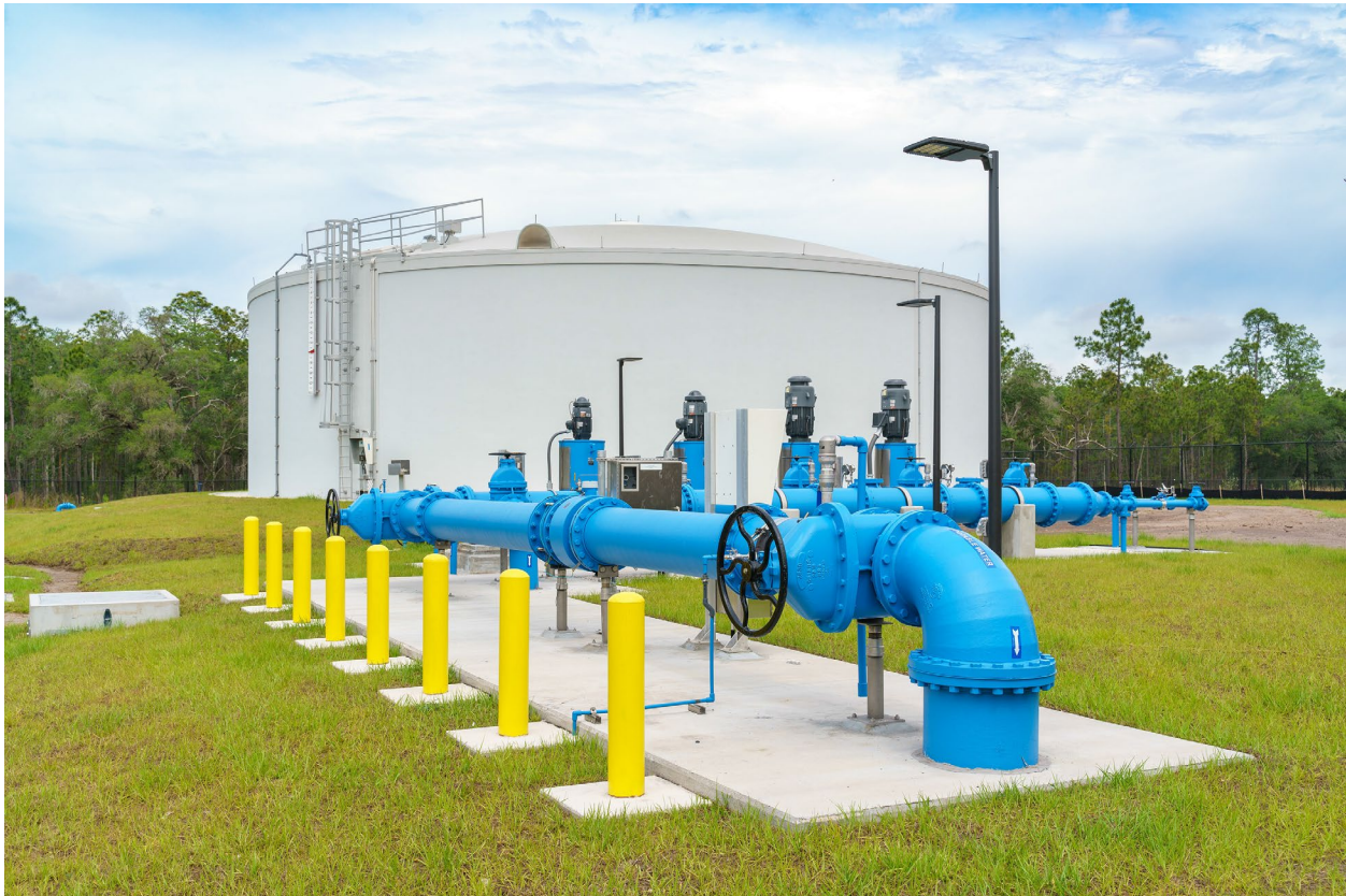
Sunbridge Water Treatment Plant
